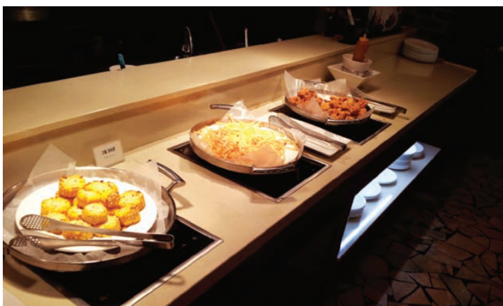
Multiple DWR04's installed with stainless steel trim in a buffet counter
